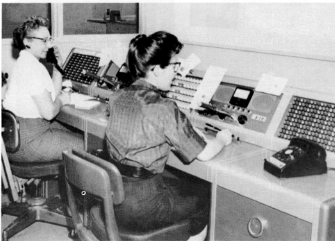
The original dispatch console with its "Christmas" light board. Red, green, and white lights indicated the status of field units.
